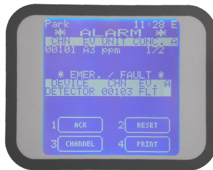
Figure 26) Active Events screen with Alarm and Fault
