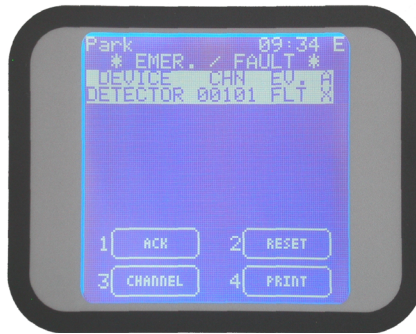
Figure 28) Active events screen with fault only
