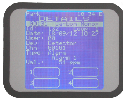
Figure 22) ALARM details screen.
